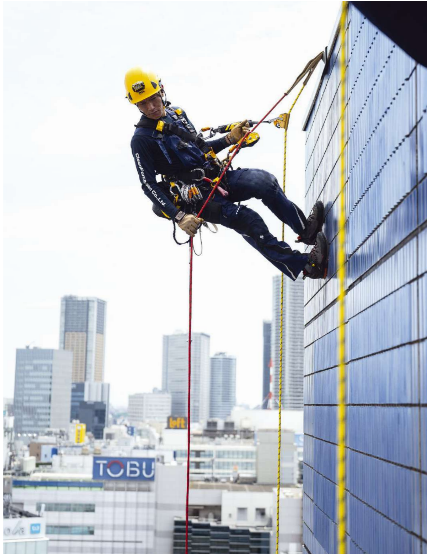
Rope access work at the Tokyo Metropolitan Theater © 2025 Petzl Distribution - Vuedici.org - Tokyo Metropolitan Theater - Clean Force Japan
